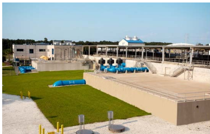
Tampa Bay Water treatment plant (Credit: Tampa Bay Water)
