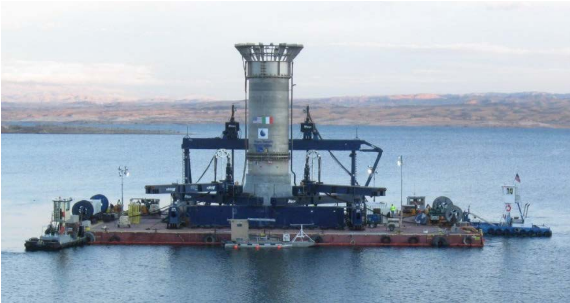
Low-level intake structure in Lake Mead (Credit: Southern Nevada Water Authority)
