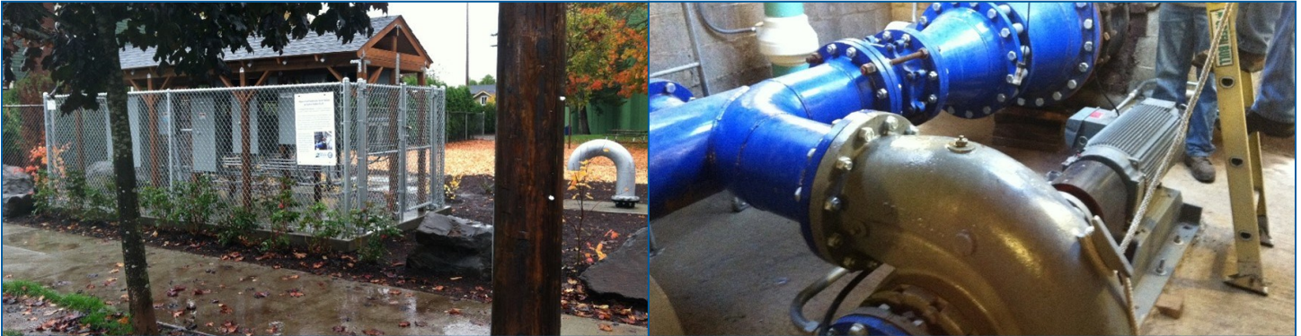
Left: Above-ground electrical invertors, drives and control equipment for inline micro-hydro
