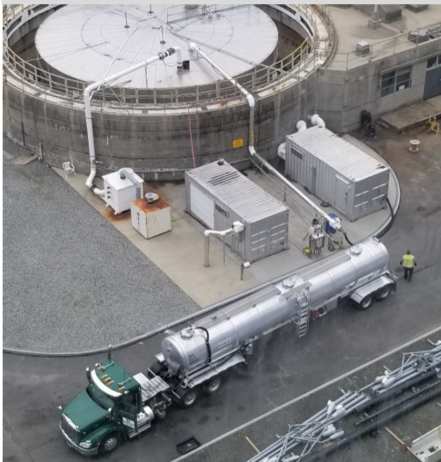
Food Waste Feed-In Station at Newtown Creek Wastewater Resource Recovery Facility Photo courtesy of Waste Management
