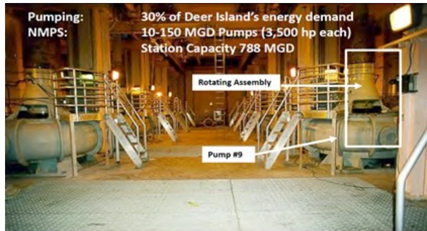
Pump #9 was operating inefficiently and was refurbished, including an epoxy resin coating on the inner shell of the pump
