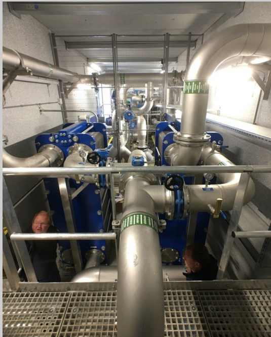
Waternet-section of the heat and cold storage installation at Sanquin Blood Bank
