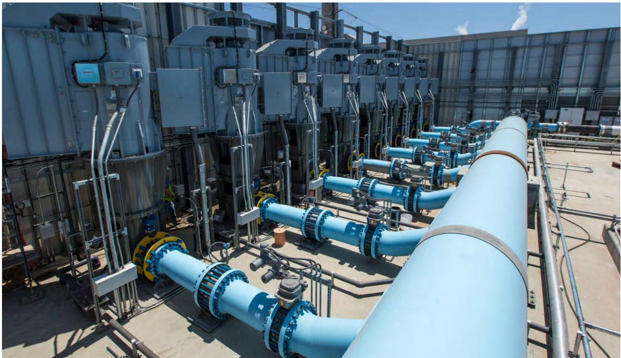
SDCWA desalination pumps and pipes
