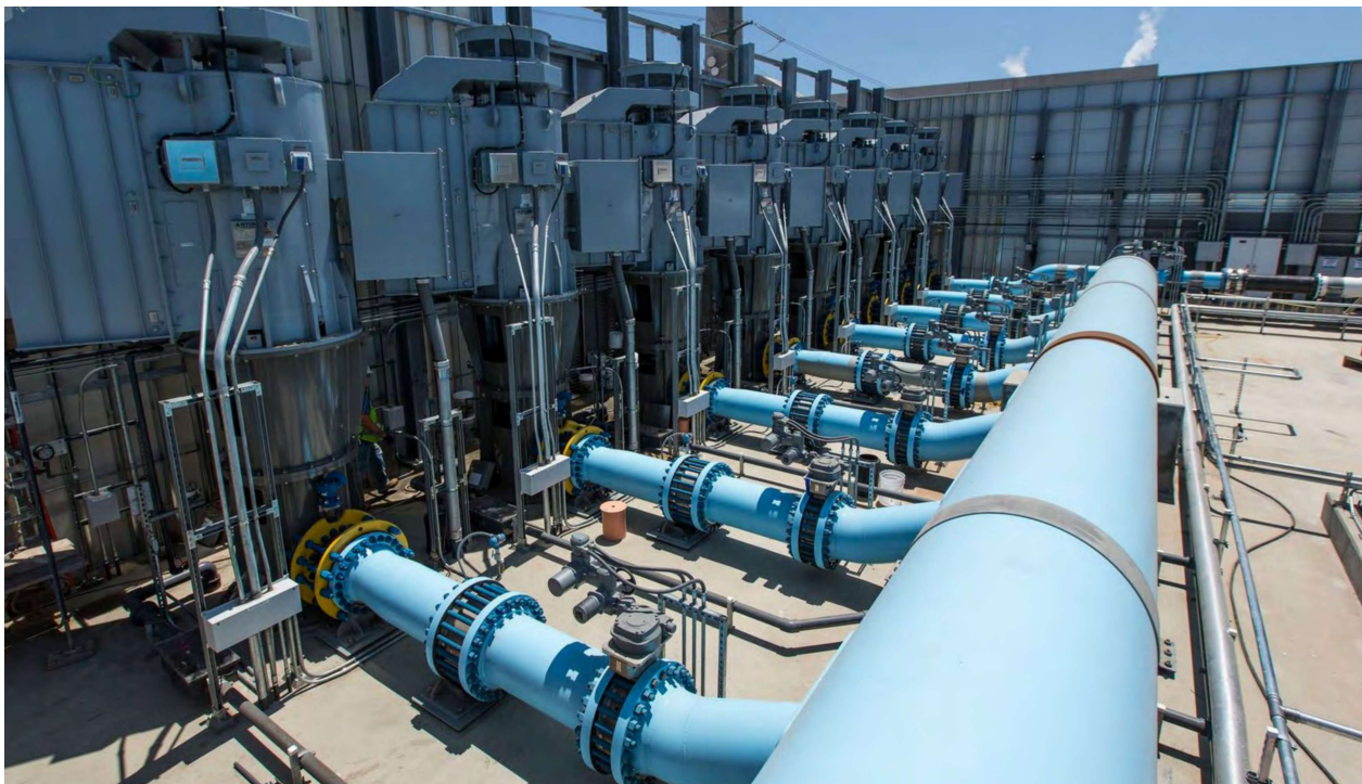
SDCWA desalination pumps and pipes
