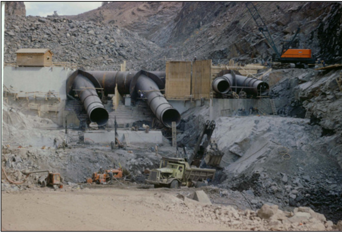
This 1964 image shows construction of the Blue Mesa Dam on the Gunnison River. (From the Ival Goslin Collection; Courtesy of Water Resources Archive, Colorado State University Libraries)
